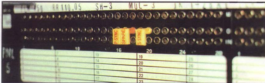
BANTAM DSX PANEL WITH I.D. PLUGS AND VARIOUS I.D. CAPS INSTALLED
