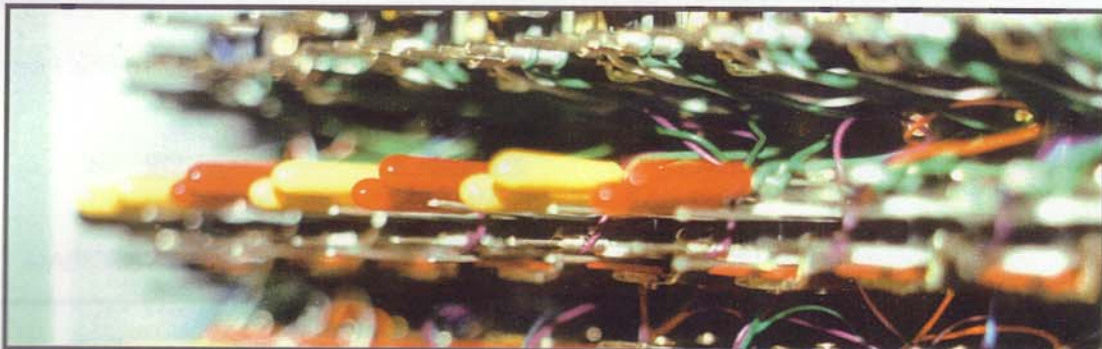
WIRE WRAP INSULATORS ON REAR OF 310 DSX PANEL INSTALLED
